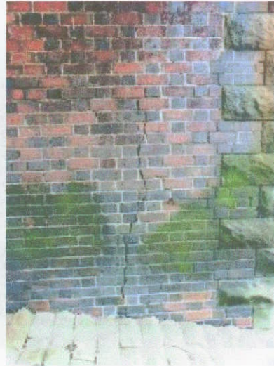
Photograph 3.92 Filey Bay 67-28B-04. Vertical crack approx. 2m high
