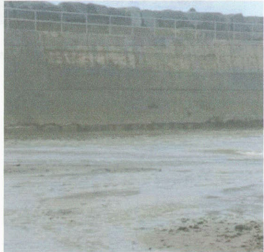
Photograph 3.6 Staithes Northern Breakwater. Abraded vertical surfaces and toe scour
