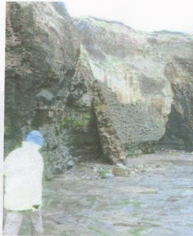
Photograph 3.42 Gouldsbrough 12-08B-01. Wash-out behind remnant seawall
