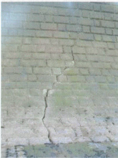
Photograph 3.60 SNB 44-20B-04 and 44-20B-03. Rocks and debris near staircase landing area
