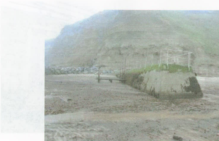
Photograph 3.18 Staithes. Concrete Pier / groyne at south-eastern corner of harbour.
