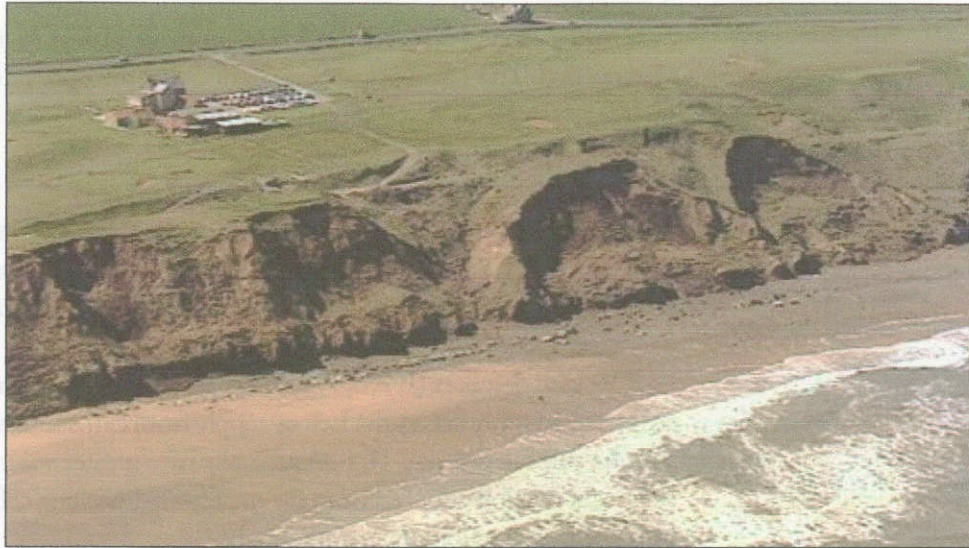
Photograph 4.5.. Undefended cliffs, Upgang Beach (profile 5 on 21/04/01 at low water +3 hrs)
