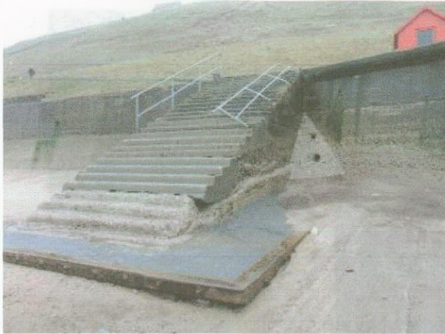
Photograph 3.55 Whitby West Cliff 20-11A-01. Loose hand railing and scour
