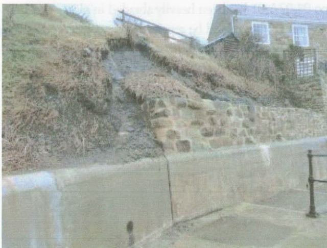
Photograph 3.35 Runswick Bay 08-07A-03. Small slip onto the upper wall at promenade level.
