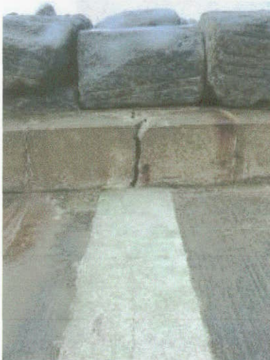
Photograph 3.5 Staithes Northern Breakwater. Abraded and damaged concrete coping
