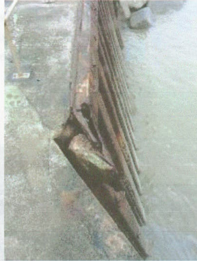
Photograph 3.4 Staithes Northern Breakwater. Corroded steel sheet piles
