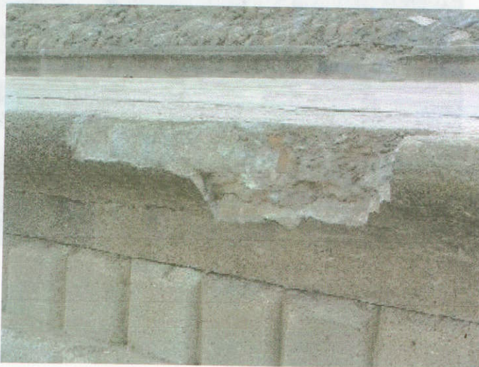
Photograph 3.70 SNB 42-20A-09. Damaged wave return wall
