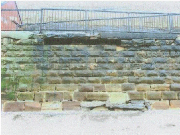
Photograph 3.57 Whitby West Cliff 20-11A-02. Masonry blocks are missing just below the promenade
