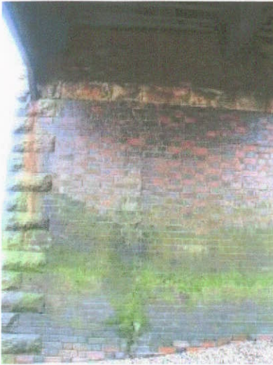
Photograph 3.91 Filey Bay 67-28B-04. Full height vertical crack
