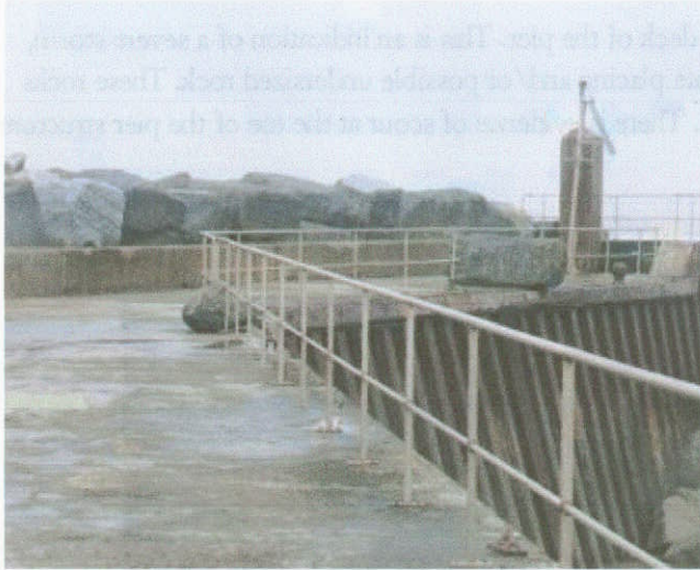
Photograph 3.3 Staithes Northern Breakwater. Displaced rock armour.
