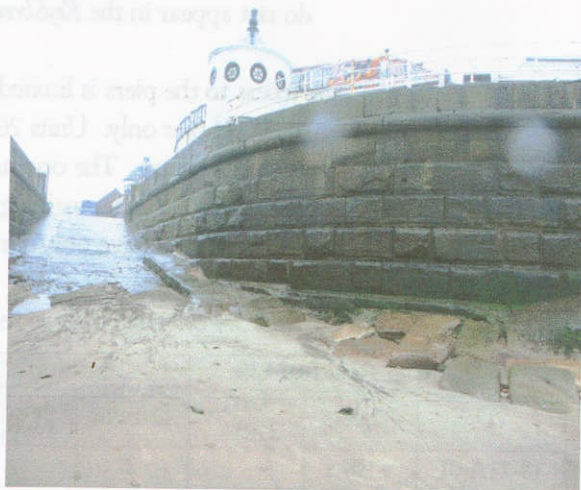
Photograph 3.62 Whitby West Pier 26-11B-02. Uneven surface at access to walkway
