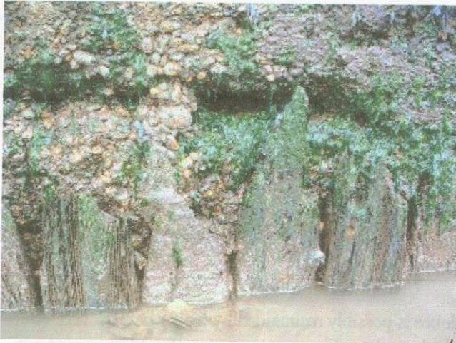
Photograph 3.76 Scarborough West Pier (SWP) Timber toe piles and localised undermining
