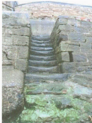
Photograph 3.34 Runswick Bay 08-07A-02. Very rounded, slippery steps
