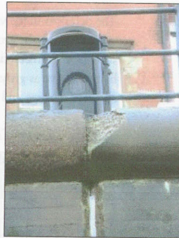
Photograph 3.48 Sandsend 14-09B-01. Minor damage to wave return feature of wall
