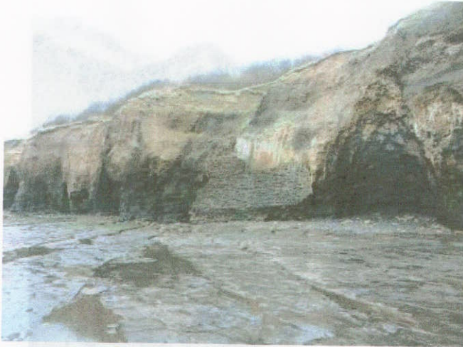
Photograph 3.41 Gouldsbrough 12-08B-01 Third remaining section of seawall
