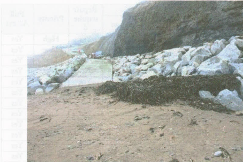
Photograph 3.64 Robin Hood's Bay (RHB) 32-16A-02. Slipway with rocks partially covering access
