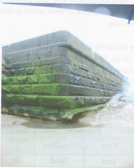
Photograph 3.61 Whitby West Pier 26-11B-02. Scour at the base of harbour wall
