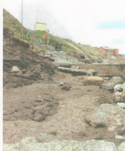
Photograph 3.88 Cayton Bay 60-24B-01. Landslip and erosion below steps
