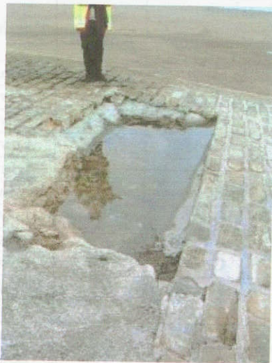
Photograph 3.74 SNB defences south of asset 44-20B-05 show some sign of wear and have suffered some damage. They require some remedial repairs
