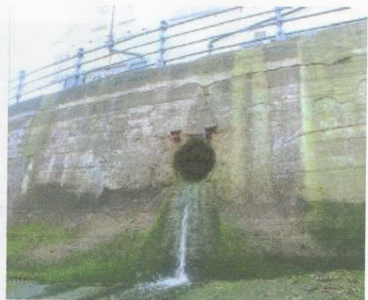
Photograph 3.15 03-04-01 Staithes. Damaged flap valves and cracked seawall.
