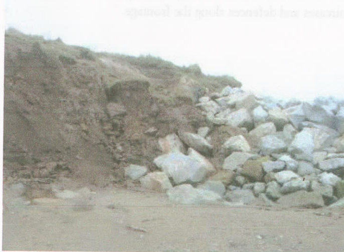
Photograph 3.67 RHB 37-16C-03. Landslip partially covering defence asset
