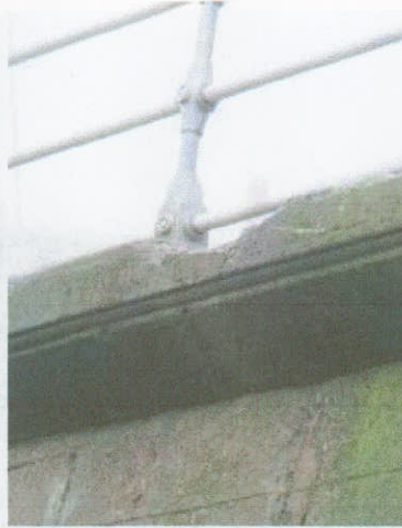
Photograph 3.56 Whitby West Cliff 19-11A-01. Damaged coping
