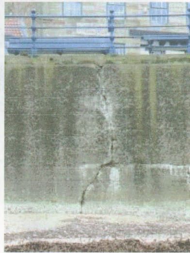
Photograph 3.17 Staithes 04-04-01 Cracked harbour walls.
