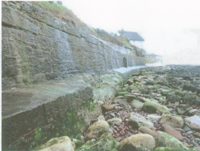
Photograph 3.33 Runswick Bay 08-07A-01. Damaged apron in front of seawall
