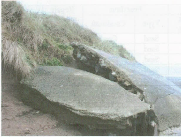
Photograph 3.51 Sandsend Wyke 17-10-01 Undermined and partially failed Defence
