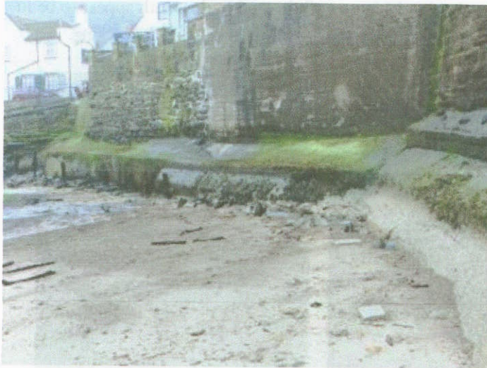
Photograph 3.12 Staithes 02-04-01. Poor condition wall, missing blocks etc
