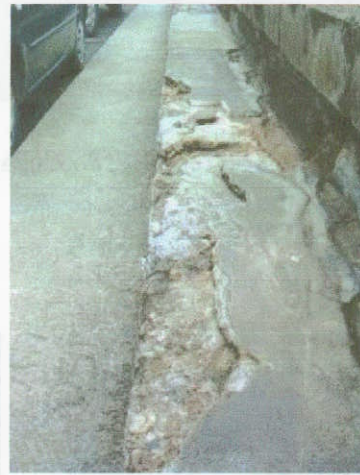
Photograph 3.83 SSB 53-22B-05. Damaged promenade kerb
