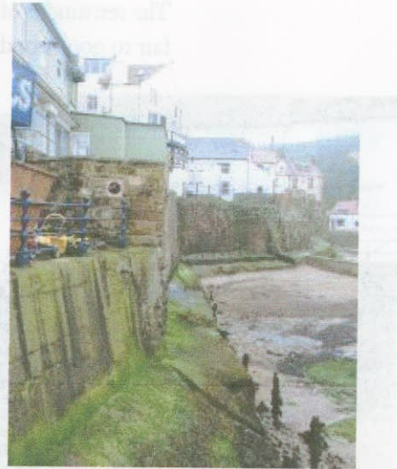
Photograph 3.13 Staithes 02-04-01. Leaning wall with toe scour.
