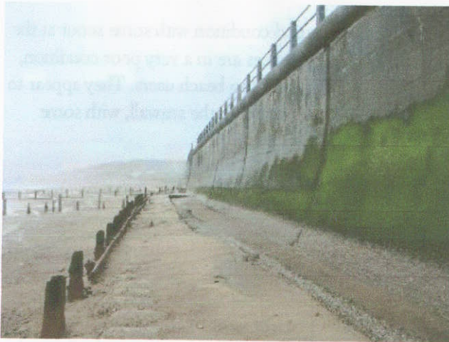
Photograph 3.47 Sandsend 14-09B-05. Light scour at toe and dilapidated groynes
