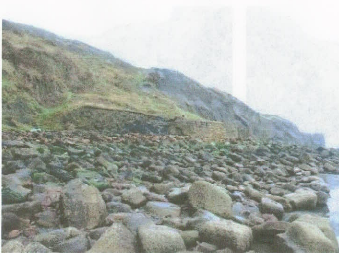
Photograph 3.43 Gouldsbrough 12-08B-01. Failed seawall with rock armour
