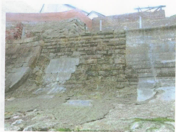
Photograph 3.86 Cayton Bay 59-24B-01. Patch repairs and interface between different wall elements
