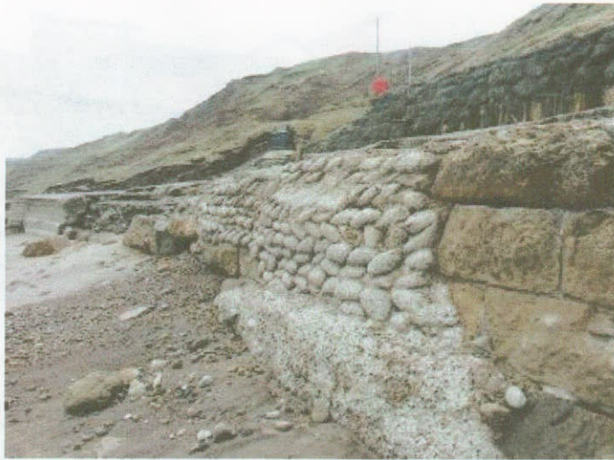
Photograph 3.87 Cayton Bay 60-24B-01. Concrete bag-work and failed defence section.
