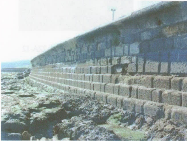
Photograph 3.82 SSB 55-22B-01. Abraded masonry blocks
