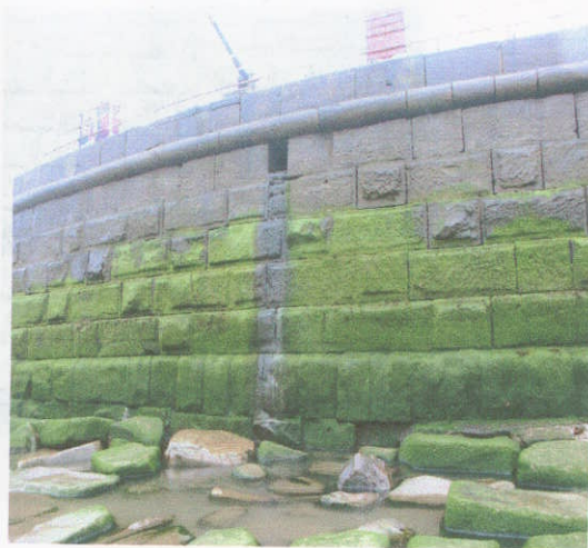
Photograph 3.60 Whitby West Pier 26-11B-01. Masonry blocks missing and surface settlement has occurred.
