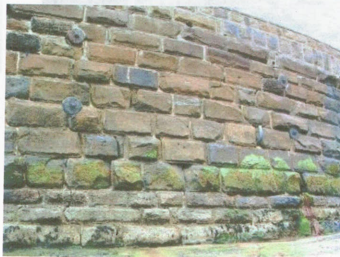
Photograph 3.81 SSB 53-22B-05. Historical cracks and anchors
