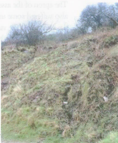
Photograph 3.36 Runswick Bay 10-07B-02. Shallow localised slope failure above the rock revetment.
