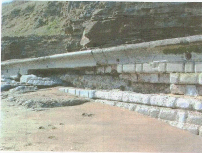
Photograph 3.84 SSB56-22B-02. Damaged and failed defences.
