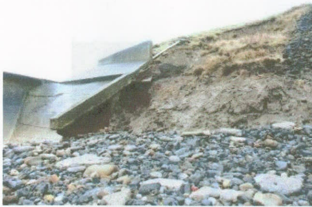
Photograph 3.49 Sandsend 13-09A-01 Undermining and erosion of defences
